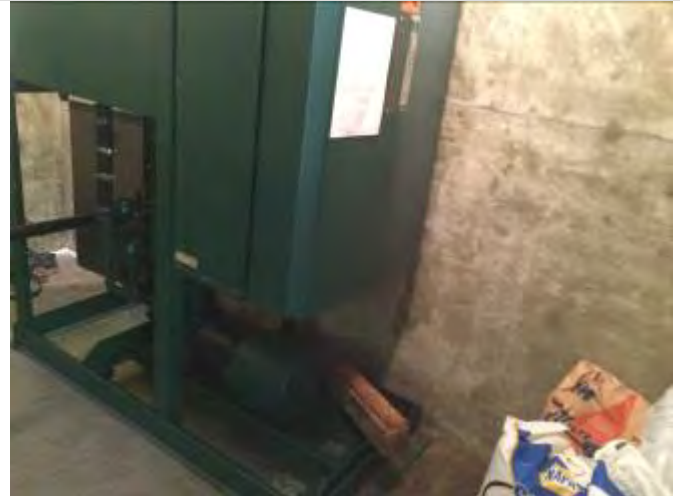
26. Hydraulic equipment for freight elevator/lift, basement
