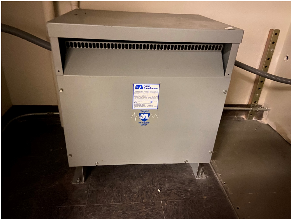
Photograph 13: Transformer in the second floor electrical room.
