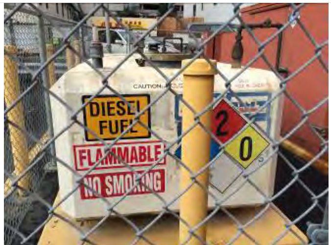
42. Alternate view of the diesel AST
