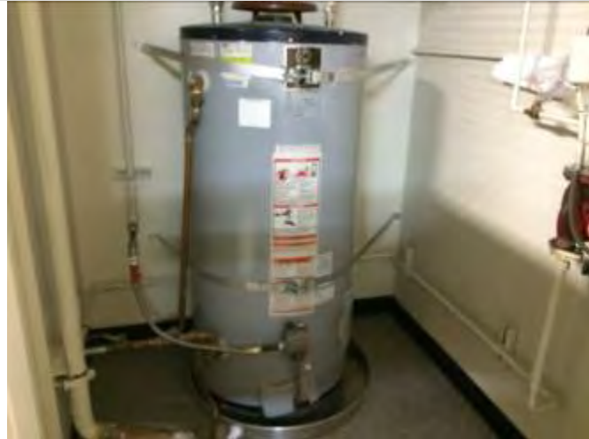
25. Water heater in restroom of Room B05
