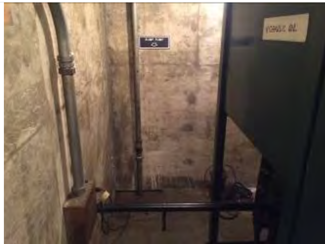
27. Sump pump behind freight elevator/lift equipment, basement
