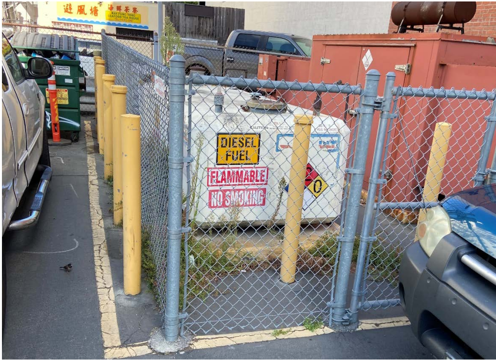
Photograph 17: Diesel-powered emergency generator in the parking lot.
