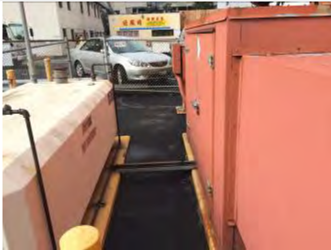
43. Aboveground piping from AST to generator
