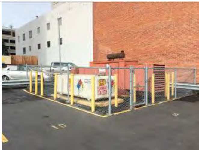
41. Back-Up Generator with above ground diesel tank and above ground piping in the parking lot
