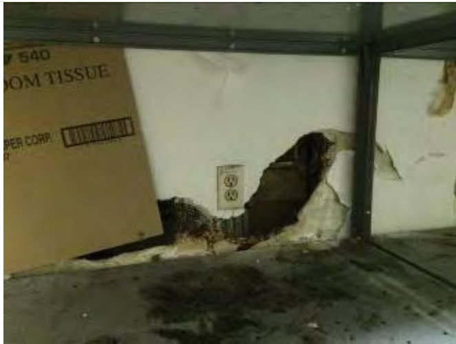
15. Damaged wallboard in basement breakroom area
