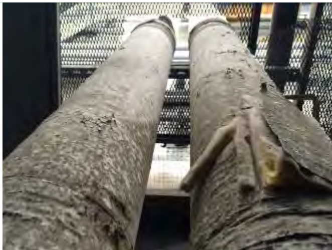
39. Fiberglass insulation on rooftop pipes
