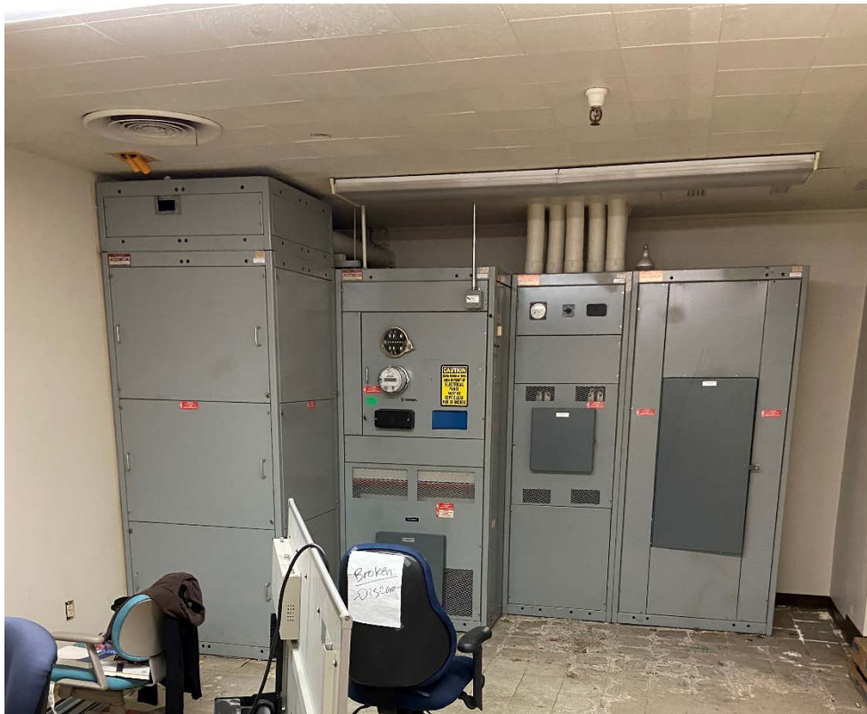
Photograph 8: Basement electrical room.
