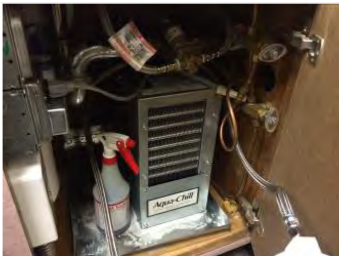
11. Under sink water filtration system in 1 st floor kitchen
