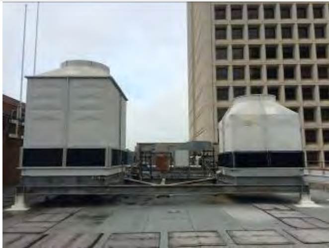
37. Rooftop HVAC equipment
