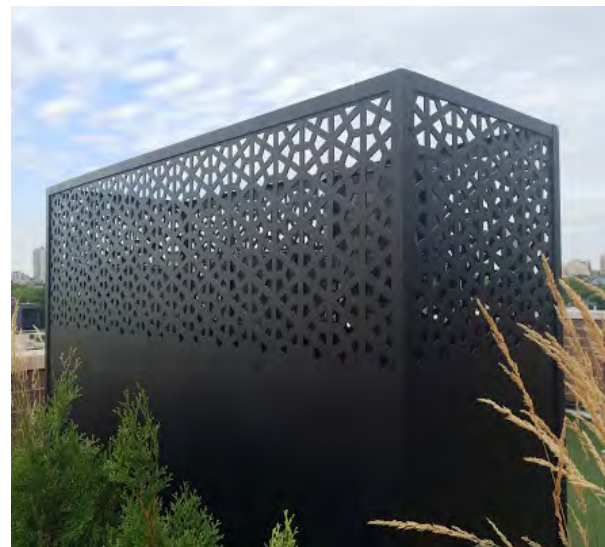
Utility decorative metal screening to shield utilities
